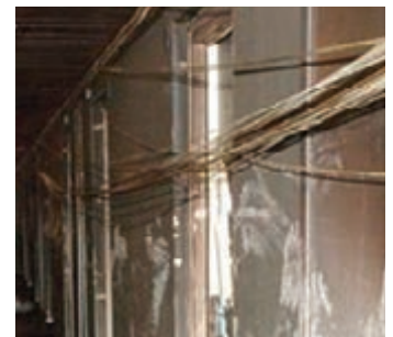
Inadequately supported cables pose risk of potentially fatal entanglements in fire conditions.
