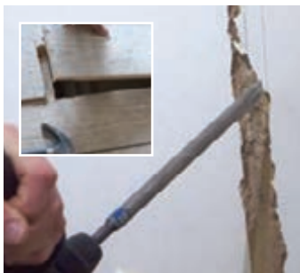
Making channels in walls, lifting floors, or using ceiling voids to hide cables can be awkward and disruptive, while repairs require co-ordination with other trades.
